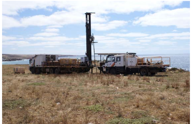
Sonic drilling rig (left) and support truck at Sheep Hill Port site in October 2008.
